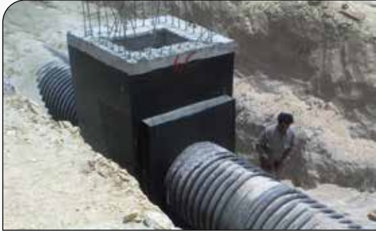
NIC HDPE Corrugated Pipes for Storm Water, connecting to Concrete Manholes at project in Kuwait
